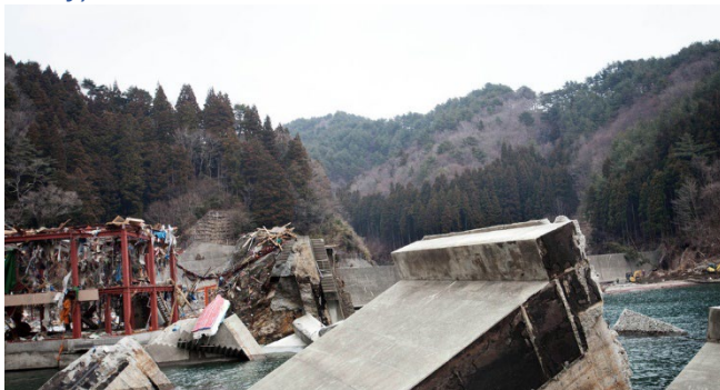
Figure 45: The Kamaishi breakwater, which failed during the 2011 Japanese tsunami (NY Times).
