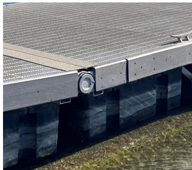
Figure 50: Example connection between boarding floats and floating tub example at the city-owned dock. (WA EMD)
