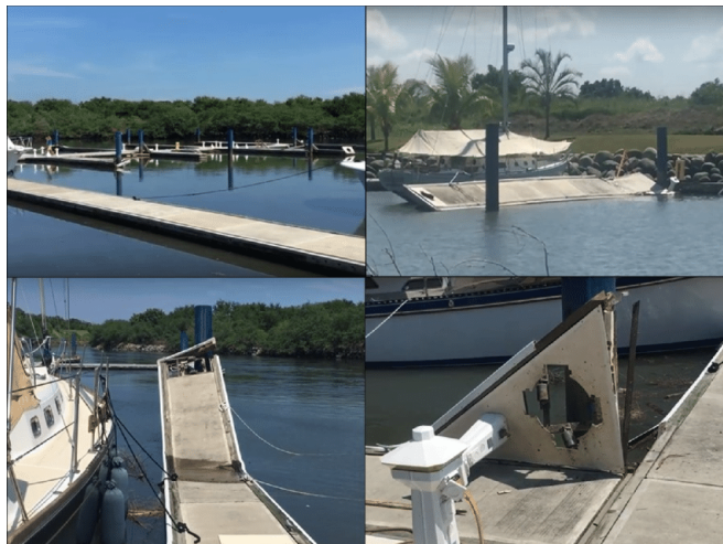
Figure 39: Dock damage in Marina Chiapas after the 2017 earthquake and tsunami. (Maria Teresa Ramirez-Herrera, 2017)
