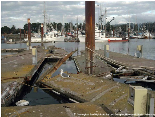
Figure 43: Broken docks in Crescent City, CA from the 2006 Kuril earthquake (USGS 2006).
