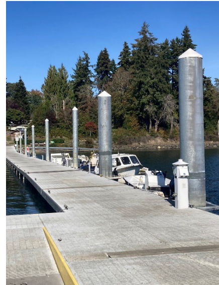
Figure 51: Pilings on the city-owned dock. Pilings further towards shore are half the diameter as the mooring pilings in the center and right of the photo (WA EMD)
