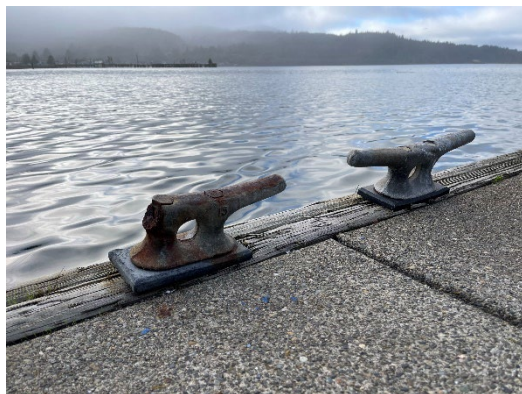
Figure 40: Broken cleat in Neah Bay along Dock A (WA EMD)
